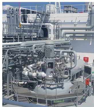
Svanehøj's cargo pumps are used for offloading liquid gas from the VLECs.
